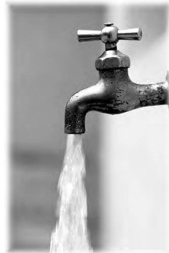
In the kitchen, check the water pressure, hot and cold water, and look for leaks.
